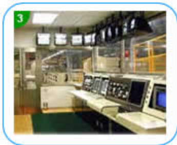
Production Control System
